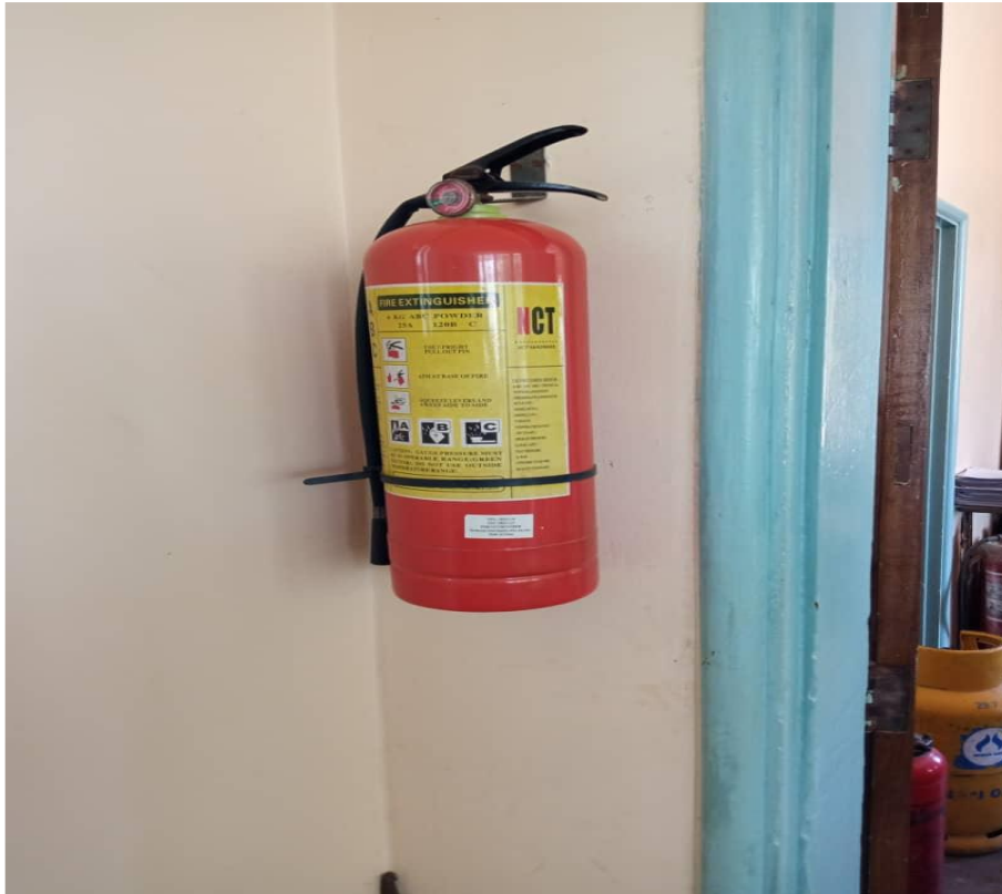
Figure 4. 1: School B's Fire Extinguisher
